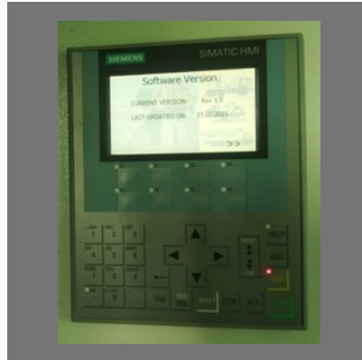
Siemens HMI for batching plant
