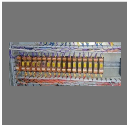
Relay For Batching Plant
