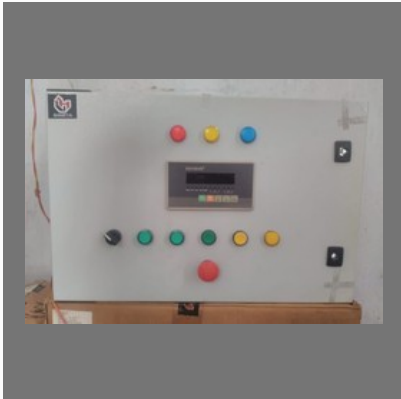
Belt conveyor panel
