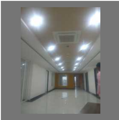
Office Interior Service
