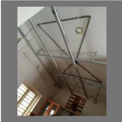
Pop Wiring Proper Fitting
