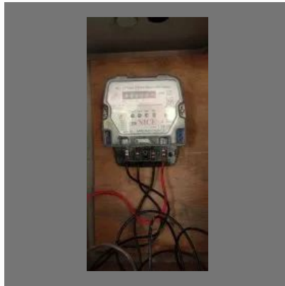
Electrical Consultation Services
