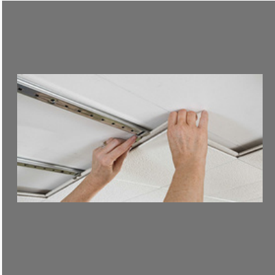
False Ceiling Services
