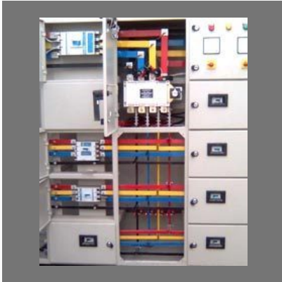
Power Distribution Panel
