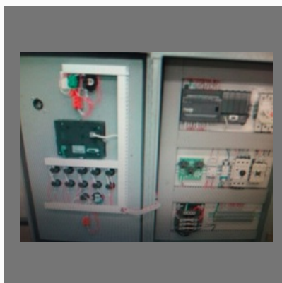
PLC Automation Control Panel
