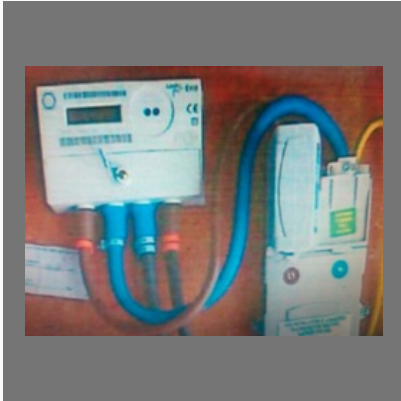
Meter Panel Board
