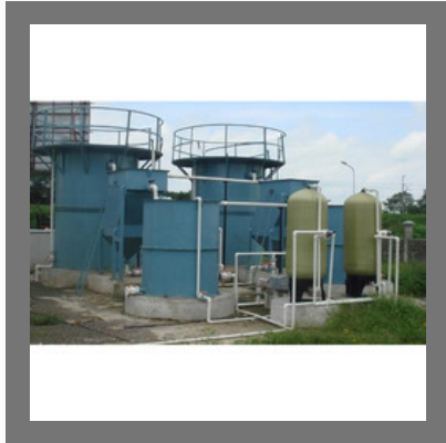
Sewage Treatment Plant
