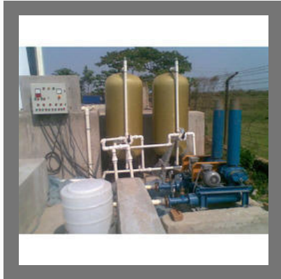
Effluent Treatment Plants
