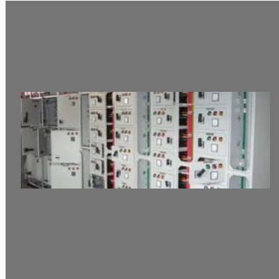
LTMV Electrical Panels
