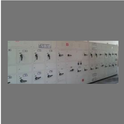
LT Electrical Panels
