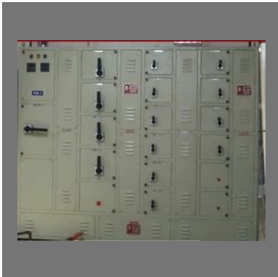
PMCC Switchgear Panel
