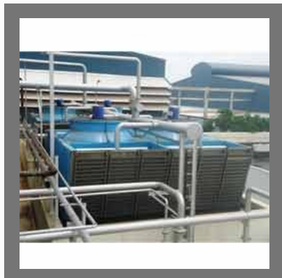
Cross Flow Cooling Tower
