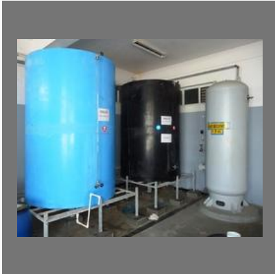
Vertical FRP Storage Tank
