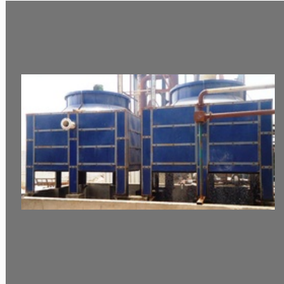
Square Shape Cooling Tower
