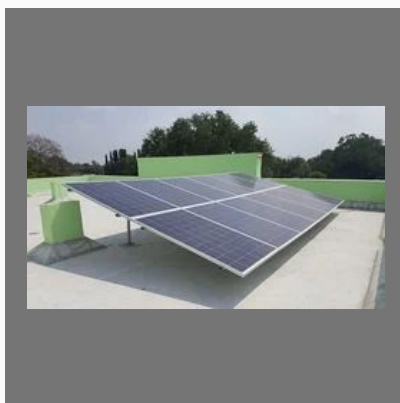
EPC Solar Power Plant
