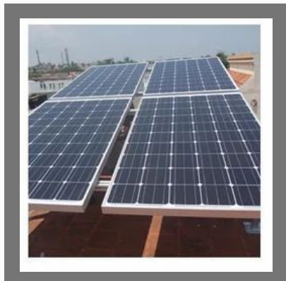
Solar Photovoltaic System
