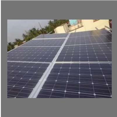
Rooftop Solar Panel
