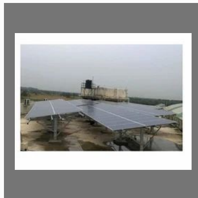
Domestic Solar System
