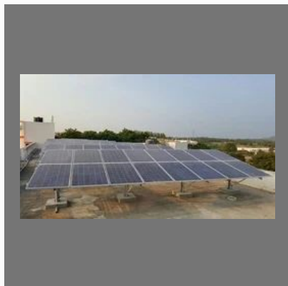
Commercial Solar System
