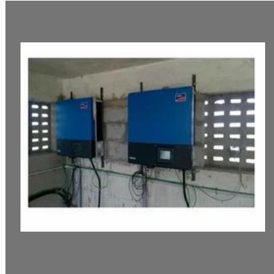
Solar Power Inverter
