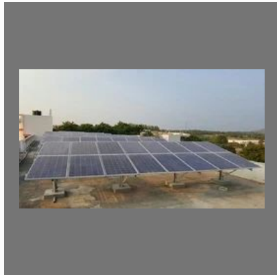
Off Grid Solar System
