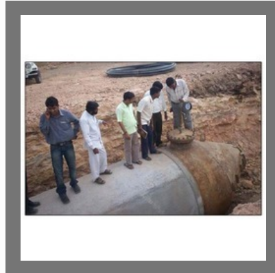
Hydrotest Inspection Service
