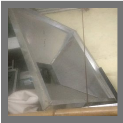
Industrial Air Duct
