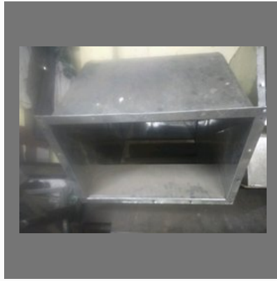
Ac Air Duct
