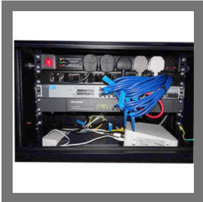
Server Networking Rack
