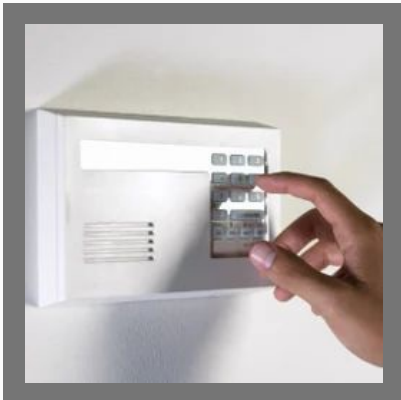
Wired Burglar Alarm Panel
