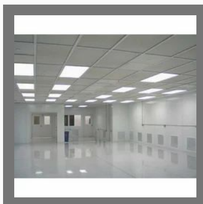
Room Panel Lighting
