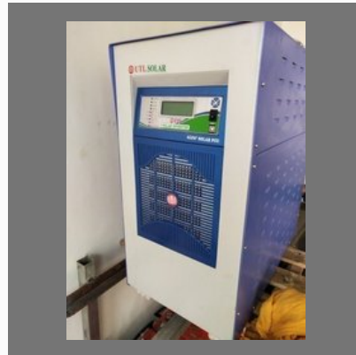
5kw Off Grid Solar System
