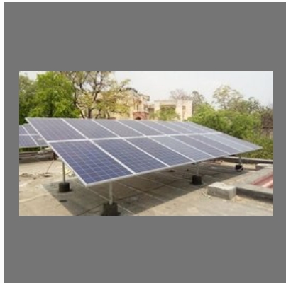
Solar Panel 12v
