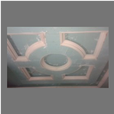
Plaster Fall Ceiling Service
