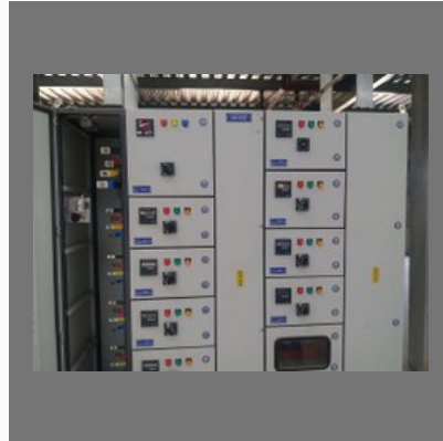
Mcc Control Panel
