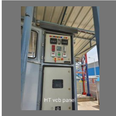
11 Kv Ht Panels
