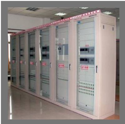
PLC Based Autoload Management
