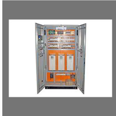
AC Drive Panel
