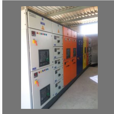
1000 kva AMF With PLC Control panel
