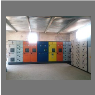
125kva AMF Panel
