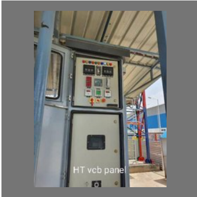
33 KV Outdoor HT Panel
