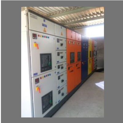
2DG Set AMF Panel
