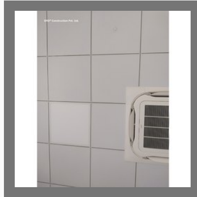
Grid False Ceiling
