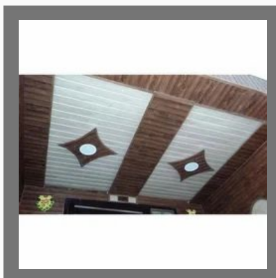
PVC False Ceiling
