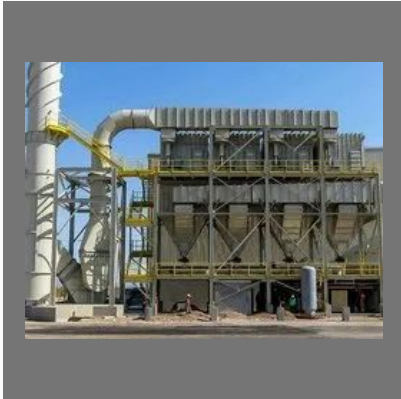
Air Pollution Control Equipment For Plant
