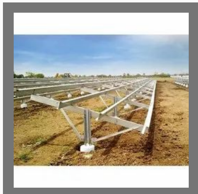
Steel Solar Panel Structure
