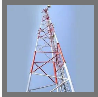
Steel Angular Telecom Tower
