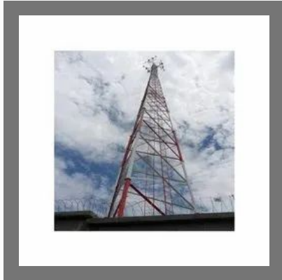
Communication Angular Tower
