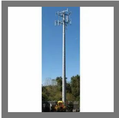
Steel Monopole Tower
