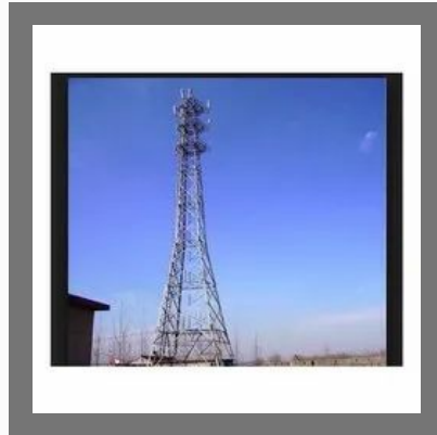
Hybrid Telecom Tower
