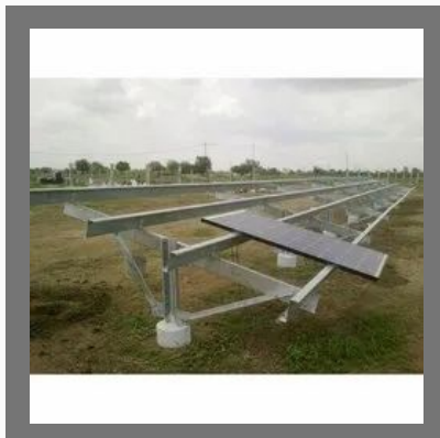
Solar Panel Structure
