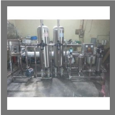
RO Plant SS
