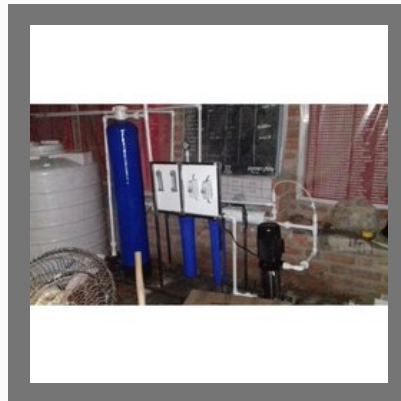
250 LPH FRP RO Plant
