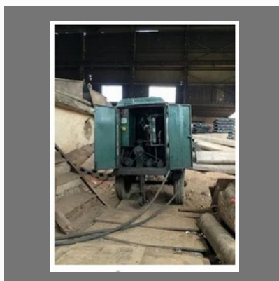
Transformer Oil Filtration
