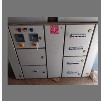
Electric Control Panel
