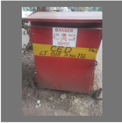
Electrical Feeder Pillars
