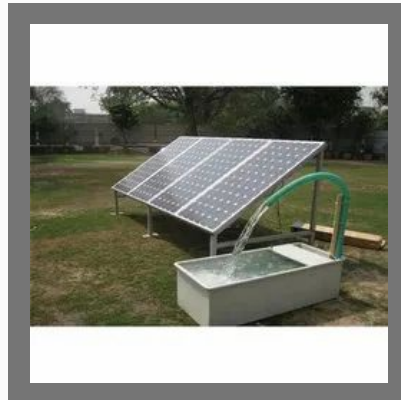
2 HP Solar Water Pump
