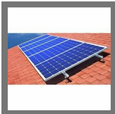
Rooftop Solar Power Panel
