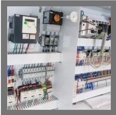
Electric Control Panel
