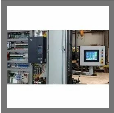
Variable Frequency Drive ( VFD )
