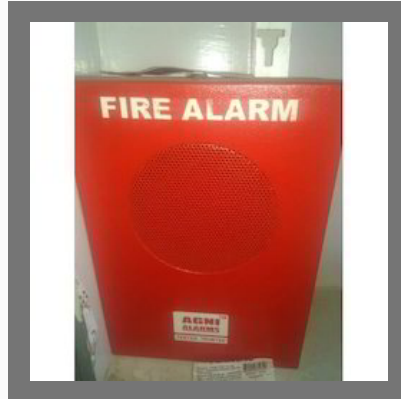
Fire Alarm System
