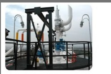
4 16 M Dia Tanks
