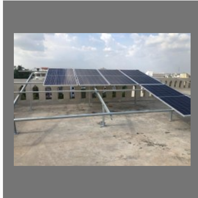
Solar Power Generation Systems
