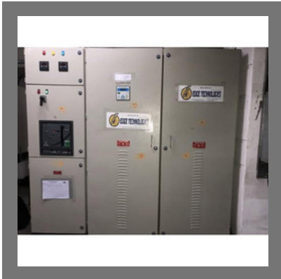
Automatic Power Factor Control Panel
