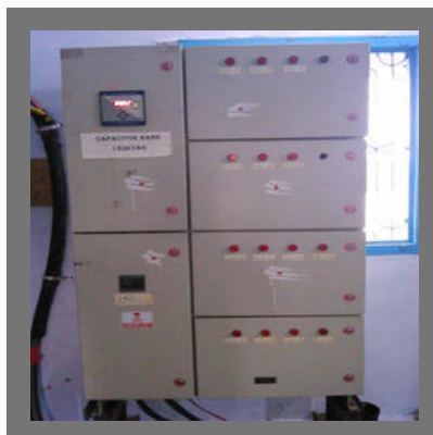
APFC Panels with Broadband Harmonic Filters
