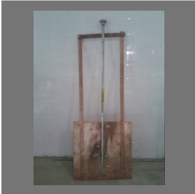
COPPER PLATE EARTHING
