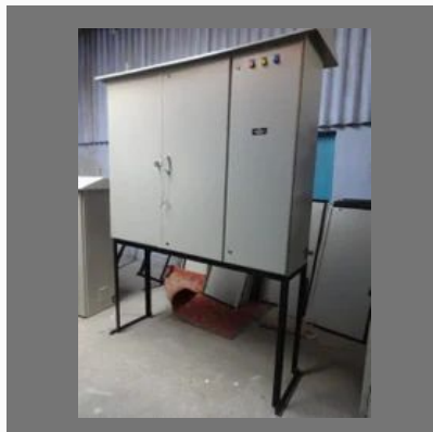
Feeder Pillar Panel
