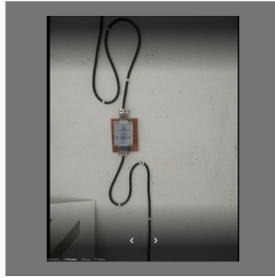
Wiring Installation Service For Commercial Plots
