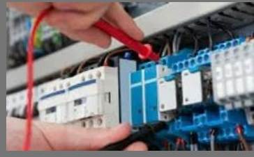
Electrical Wiring Service
