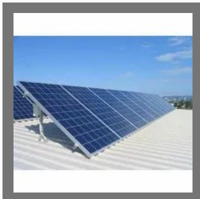
7.5 kW Off Grid Solar Power Plant
