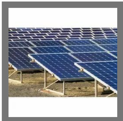
7.5 kW On Grid Solar Power Plant
