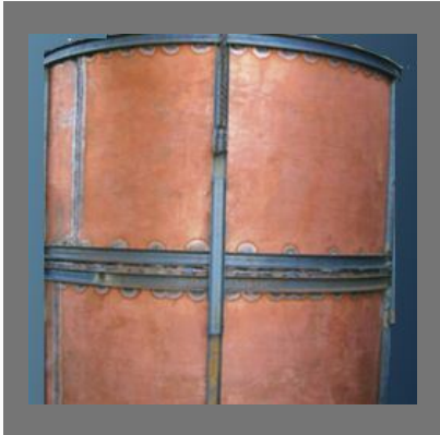
Fuel Storage Tanks
