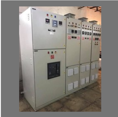
Real Time Power Factor Correction Panel
