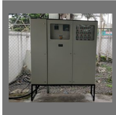
Automatic Power Factor Control Panel
