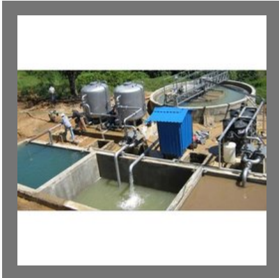
Effluent Treatment And Wastewater Treatment Plant
