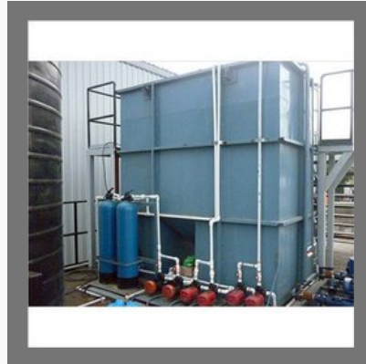
Packaged Sewage Treatment Plant
