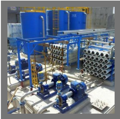
Industrial Water Treatment Plant
