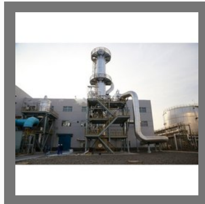
Zero Liquid Discharge System
