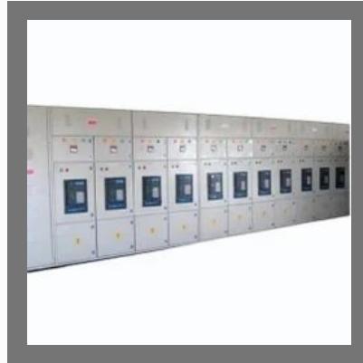
Power Control Center Panels
