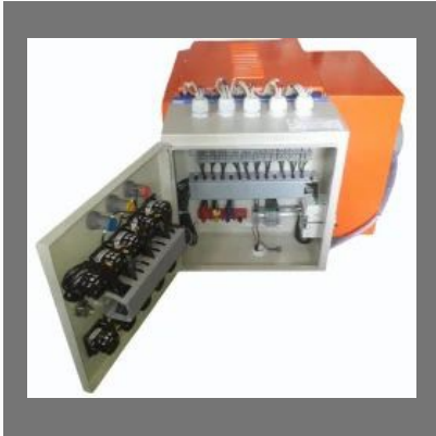
1000 kW Resistive Load Bank
