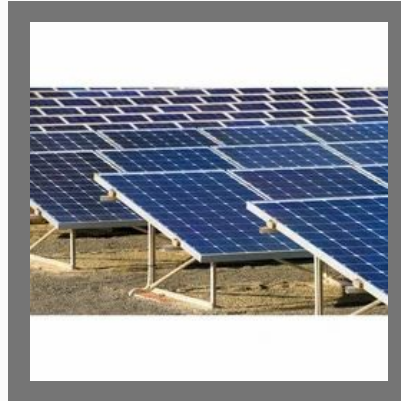
Industrial Solar Power Plant
