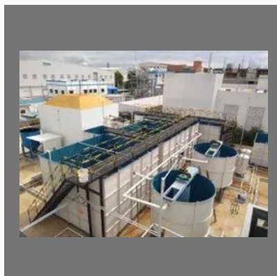
Effluent Treatment Plant With R.o System
