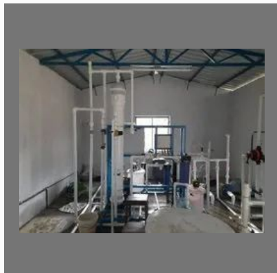
Sewage Treatment Plant With UF System
