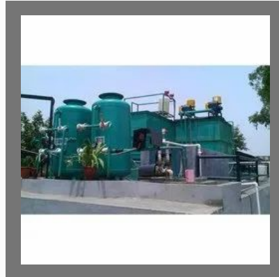
Sewage Treatment Plant With MBBR Technology
