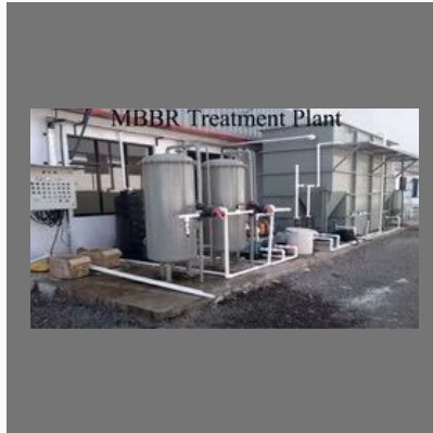
Dairy Effluent Treatment Plant
