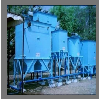
Effluent Treatment Plant Service
