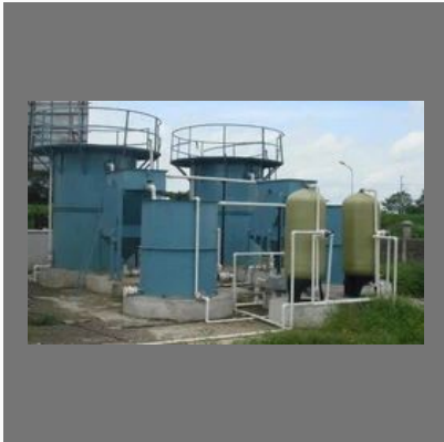
Effluent Treatment Plant Services
