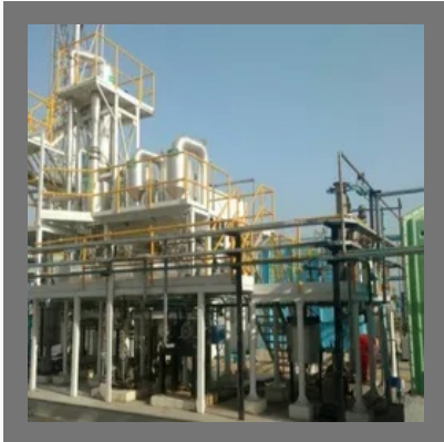
Zero Liquid Discharge System
