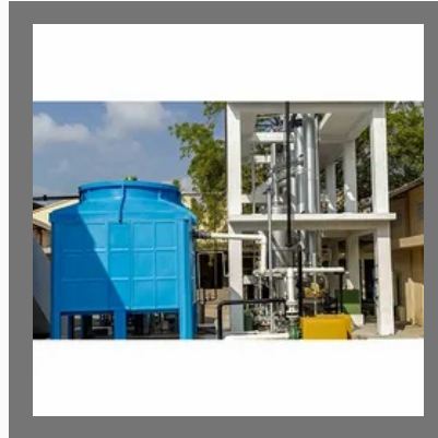
Containerized Effluent Treatment Plant
