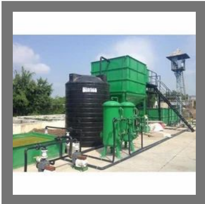
STP With SBR Technology
