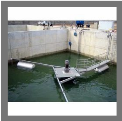
ETP Operation Services
