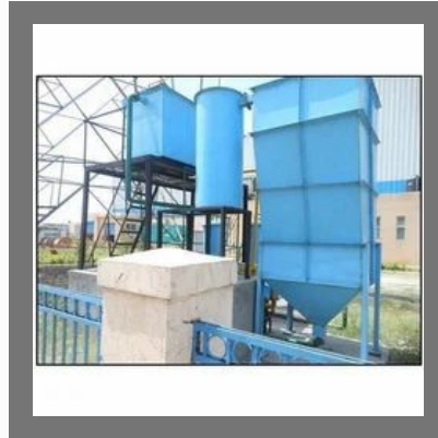
Effluent Treatment Plant
