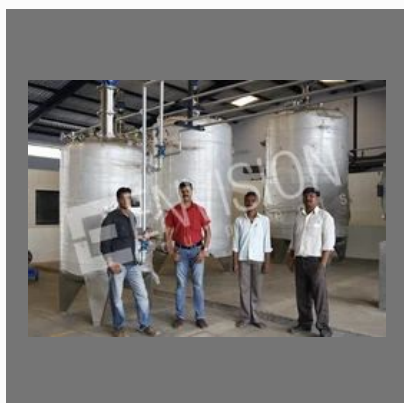
Chemical Storage Tank
