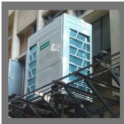
VRF Air Conditioning System
