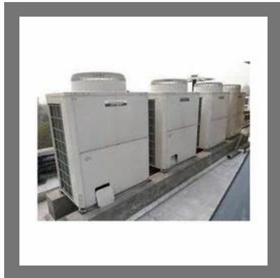
VRF Air Conditioning System
