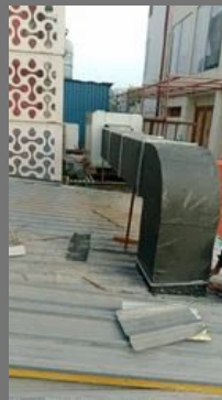
Hvac Ducting Contractor
