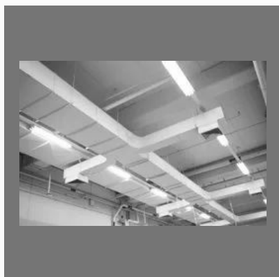
Rectangular Ceiling Mounted Air Duct
