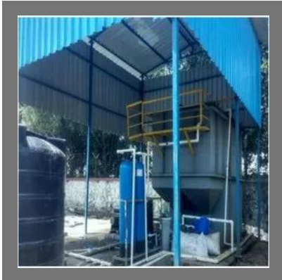
ETP Effluent Treatment Plants
