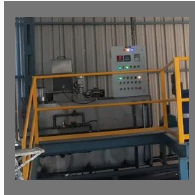
Automatic Polyelectrolyte Dosing System
