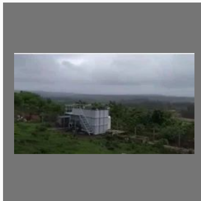
Sewage Effluent Treatment Plant STP
