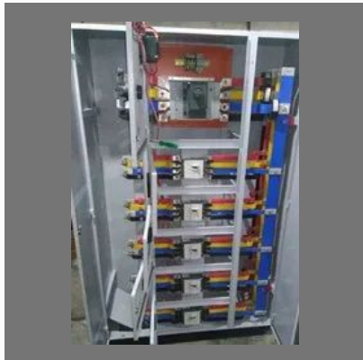
Solar ACDB Distribution Box
