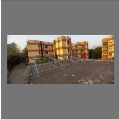
Rooftop Solar System
