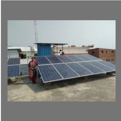
Vikram Solar Panels
