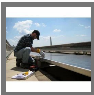
Solar Panel AMC Service
