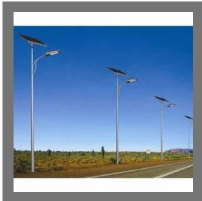
Solar Highway Street Light
