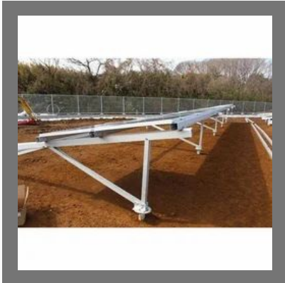
Solar Ground Mounted Structure
