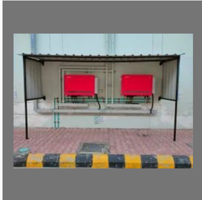
Solar Power Plant
