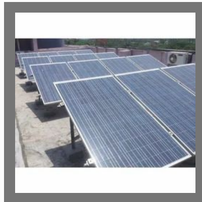
Solar On Grid Power Plant 10kWp
