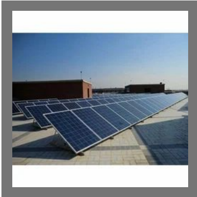
Solar Rooftop Power Plant
