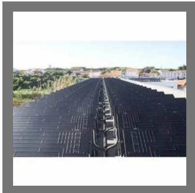
Solar Water Heater(FPC)
