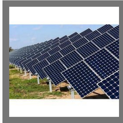
Solar Power Plant
