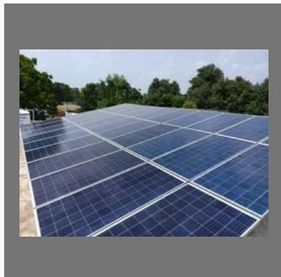
Solar Power Plant
