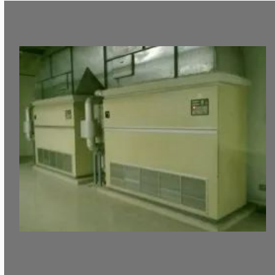
Commercial Office AC Repair And Service
