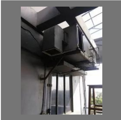
Centralized AC Repair and Service
