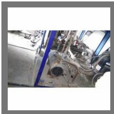
Chiller Maintenance Service
