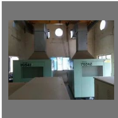
Commercial AC Unit Repair And Service
