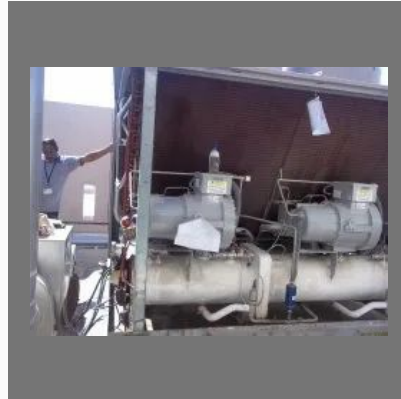
Screw Chiller Maintenance Service
