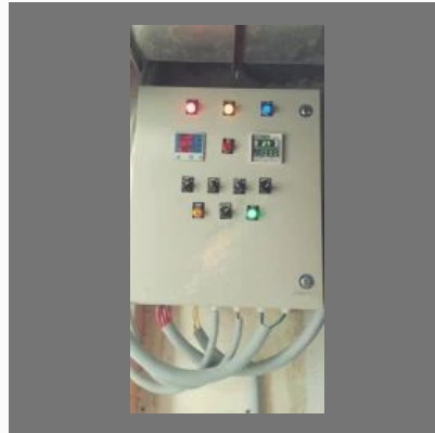
Carrier Package Ac Repair and Service
