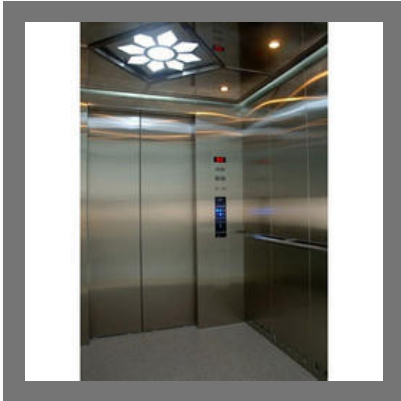
SS Elevator Cabin
