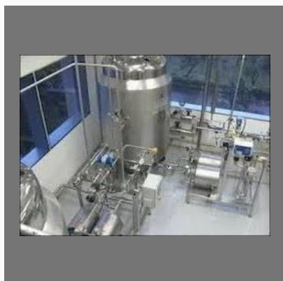
WFI Distribution Loop System
