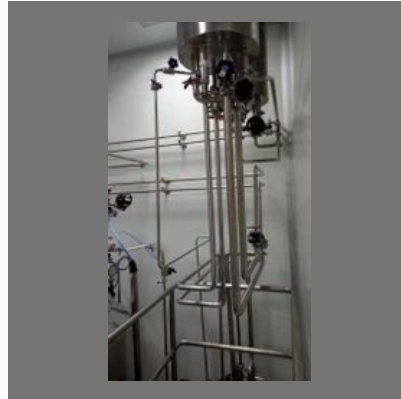
SS Process Piping
