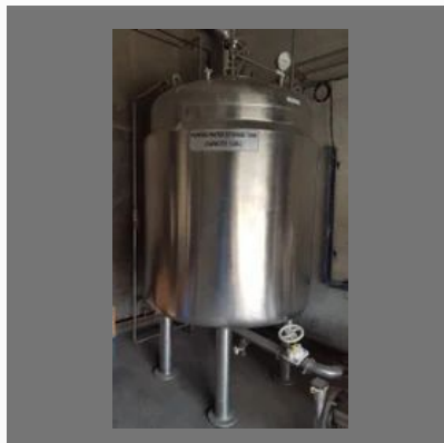
Purified Water Storage Tank
