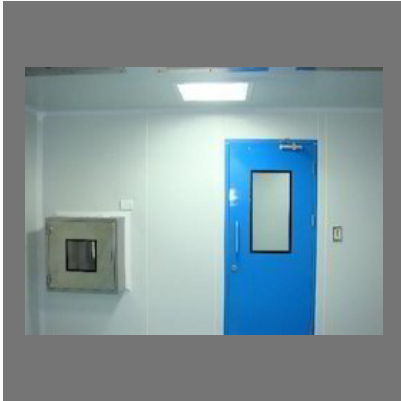
Clean Room Pass Boxes
