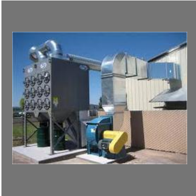
Turnkey Dust Collection System
